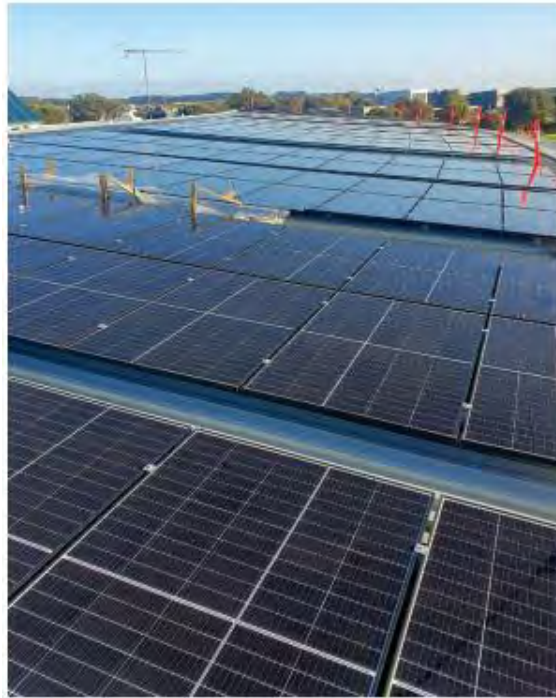
Figure 9. 100kW solar panel system has been installed on the clubhouse roof at The Sands Torquay, along with a 50kWh battery to capture excess energy for the local community.
